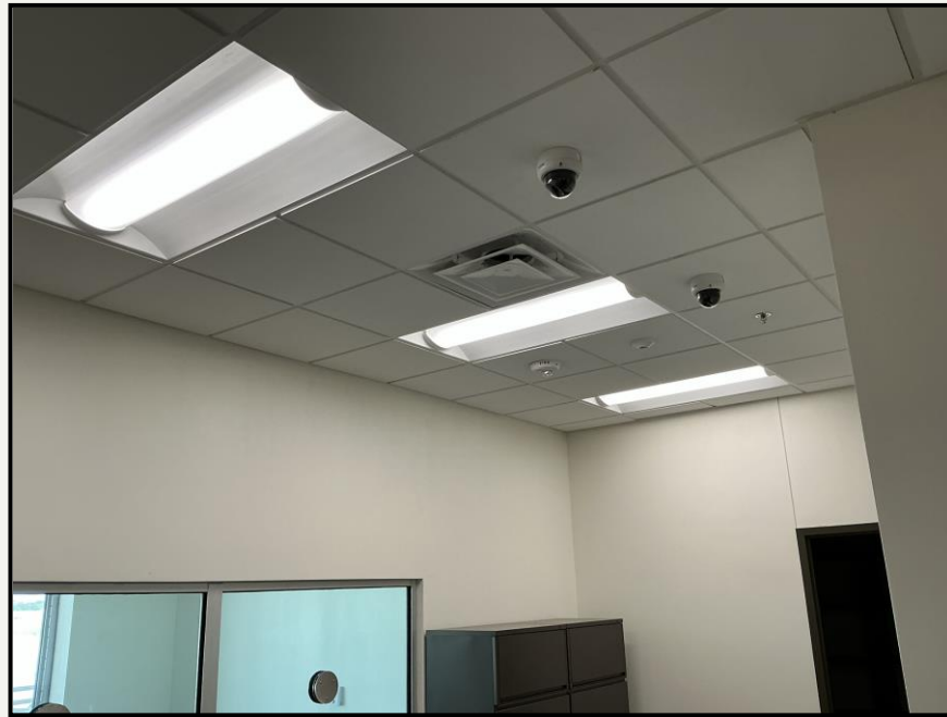
Outbound Administration Building Monitoring Equipment
