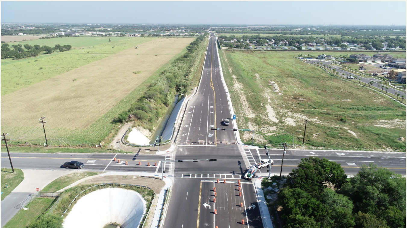
Freddy Gonzalez Dr. – Completion pending construction of HCWID No.1 infrastructure, replacement of broken inlet tops and failed concrete sidewalk replacement.
